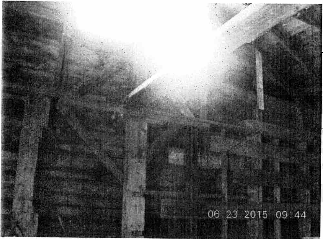
WINDOW FALLING OUT DUE TO BOWED GABLE WALL
