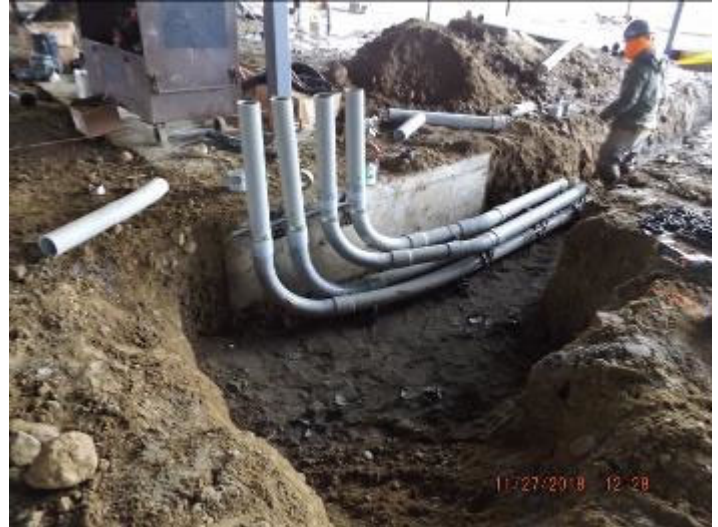
Photo depicts the installation of the primary electrical conduits into the building.
