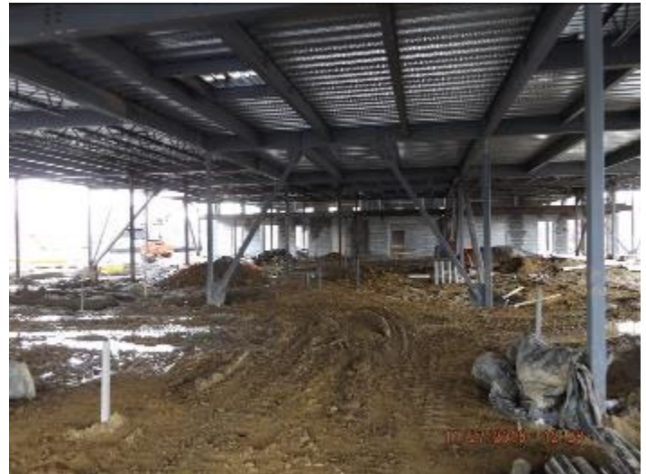
Photo depicts the installation of underground plumbing and electrical on police side.
