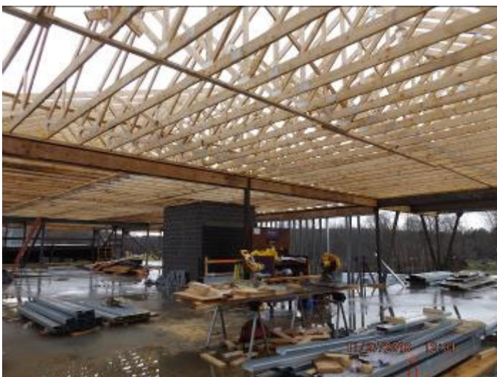
Photo depicts the installation of roof trusses, and start of metal framing on the second floor.
