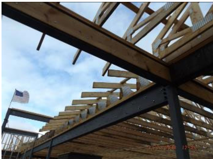
Photo depicts the detail of the blocking bolted connections for the roof trusses.
