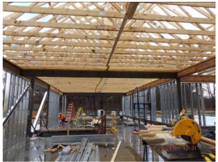
Photo depicts the installation of roof trusses, and start of metal framing on second floor.
