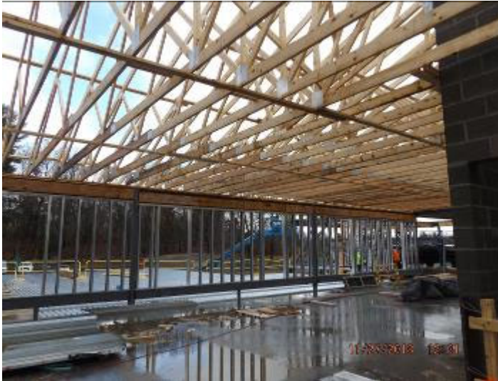
Photo depicts the installation of the roof trusses, and start of metal framing on the second floor.
