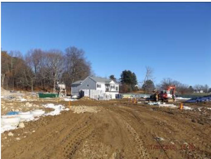
Photo depicts the completion of the water line and site drainage on the apparatus bay side.
